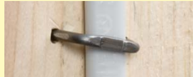
Hammering electrical cable staples too tightly into studs during rough wiring
