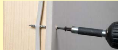
Accidentally piercing electrical cable behind drywalls with drill bit, nail, or screw
