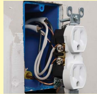
Screw terminal where a wire is connected to a receptacle may become loose as it is pushed back into the work box
